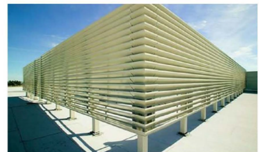
5. PENTHOUSE EQUIPMENT - SCREEN
